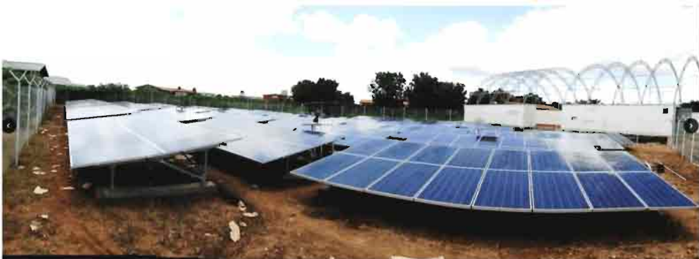
Figure 65. Solar panels in the University of Juba, South Sudan
