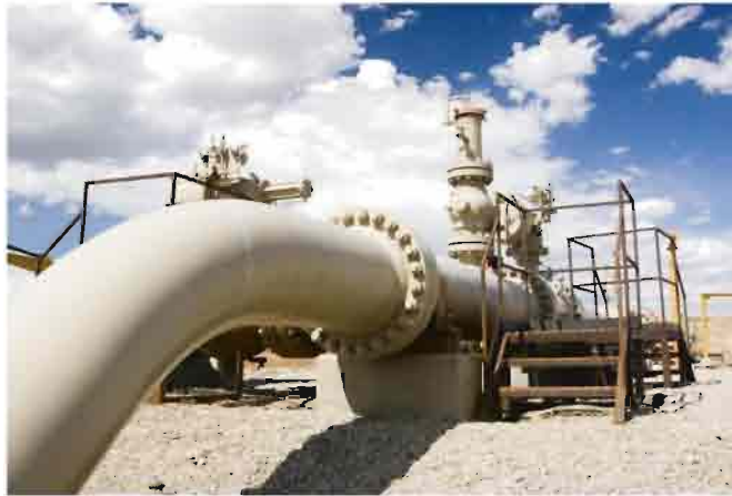
Figure 63. An oil pipeline at Gumry Oil field, South Sudan.
