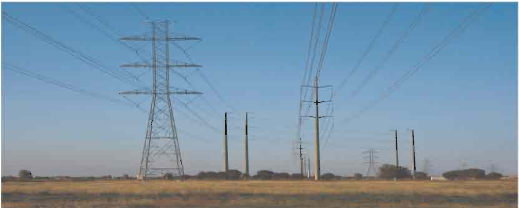
Fig. 8.1: Pylons and electricity transmission cables
