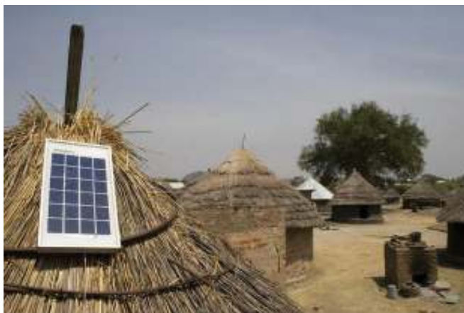
Solar panel on a roof top in a village.
