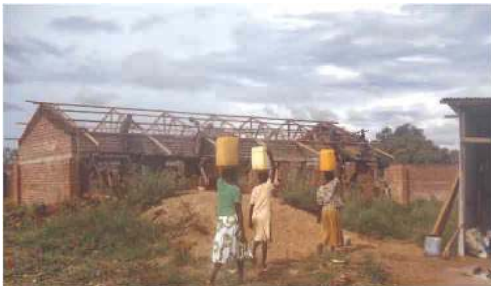
School construction project. This is an example of social impacts of a project.
