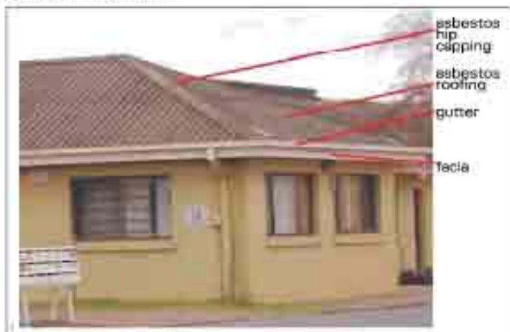
A house with asbestos roofing material.
